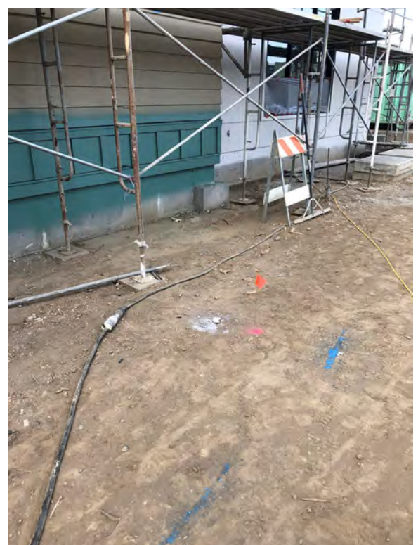
Eastern Side of Central Portion of MVHS Facing North – Sampling Location BP-43
